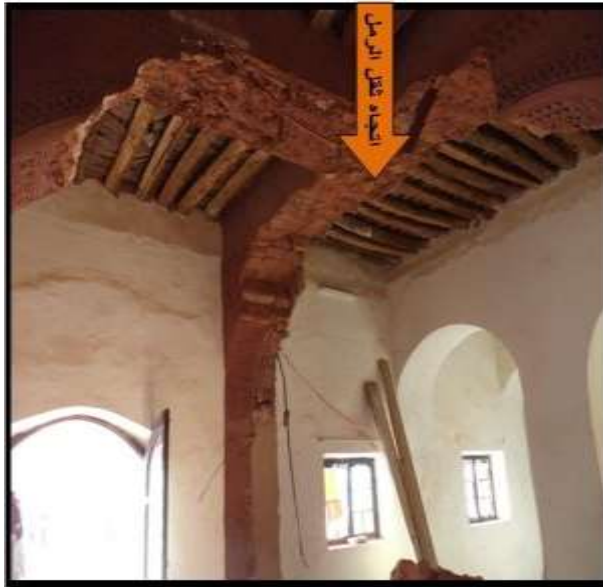
Figure 15: Image showing the collapse of the support for the three arches due to the removal of the wall.
